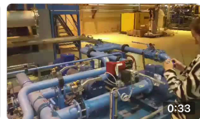
Very loud! The LHC cooling systems compressors. 8 years ago · 303 views 16
